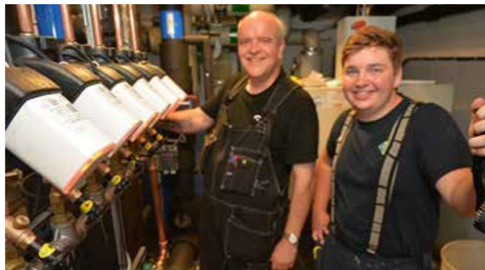
The sanitary fitters Roland Haubold and Ken Mothes from GK Pipes in Moss installed both systems here in the Orkerød Nursing Home.
