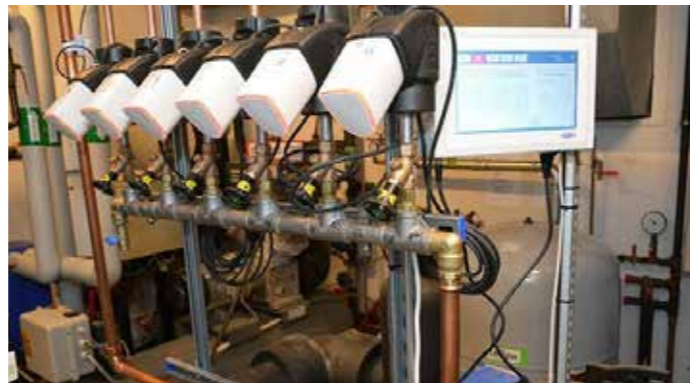
Sensors/valves have been installed on each hot water routing at Orkerød Nursing Home, shown here in the control room. On the right is the touch screen for the system.
