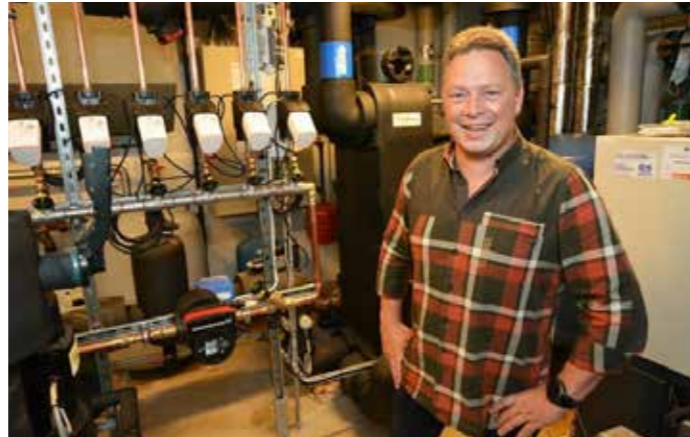
Daniel Mothes of the Moss Kommunale Eiendomsselskap (Moss Municipal Real-estate Company) has been the driver behind the installation of the system.
